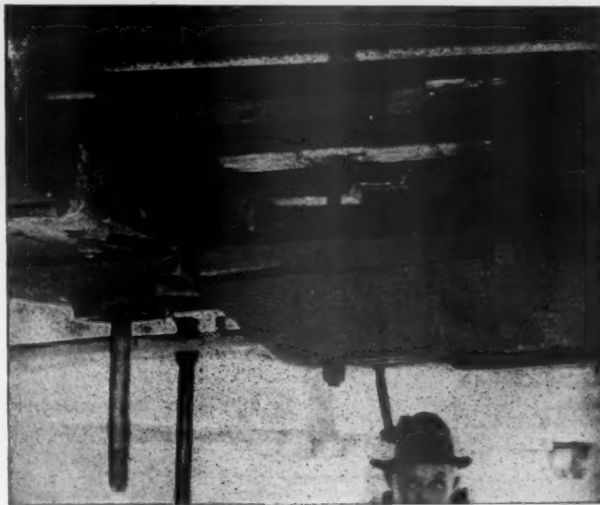
Fig. 2—One of the Common Failures.
